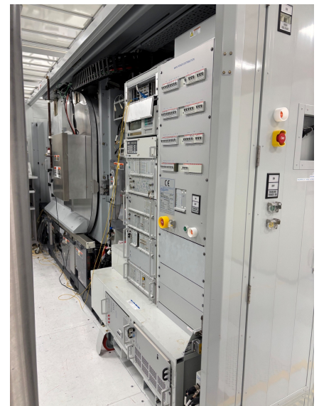
Power distribution and control racks, CE-marked
